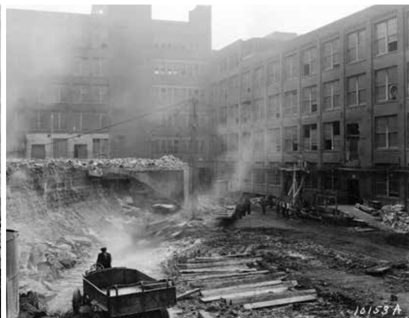
LEFT: Breaking ground on the new Federal Reserve Bank of Cleveland building.
